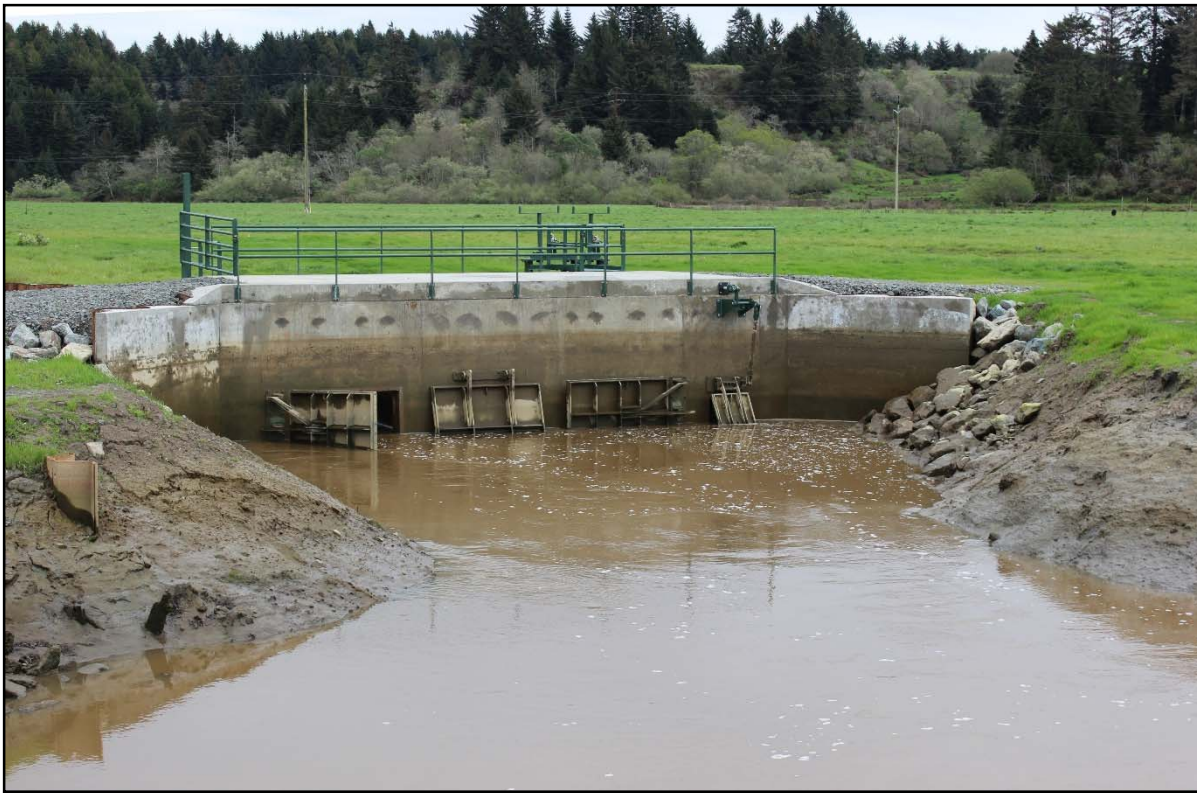
Martin Slough Tide gates, downstream side, showing the three 6' x 6' gates on the center and left and the 2' x 2' "habitat door" on the right.
