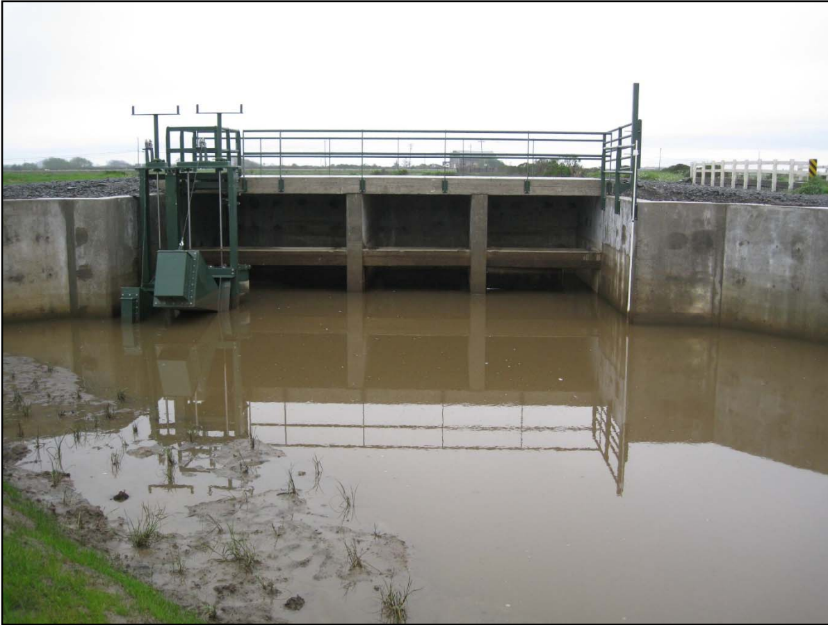
Martin Slough Tide gates, upstream side, showing the two MTR floats at left
